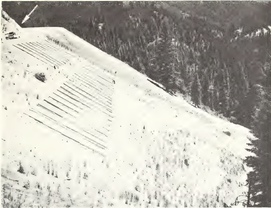
Figure 2.--The study site on a road fill approximately 200 feet long on the Deadwood River Road. Arrow points to vehicle, which provides a perspective of the size of the road fill. (Photo taken May 1968.)
